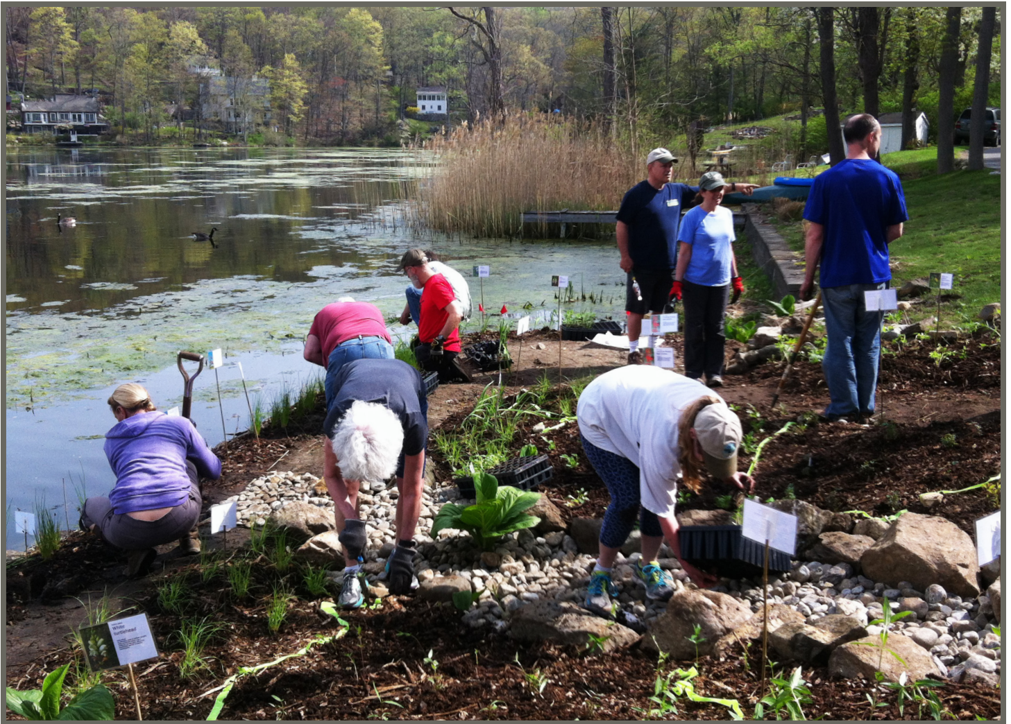
A team of volunteers helps to install a riparian buffer system on the lake association's property.
